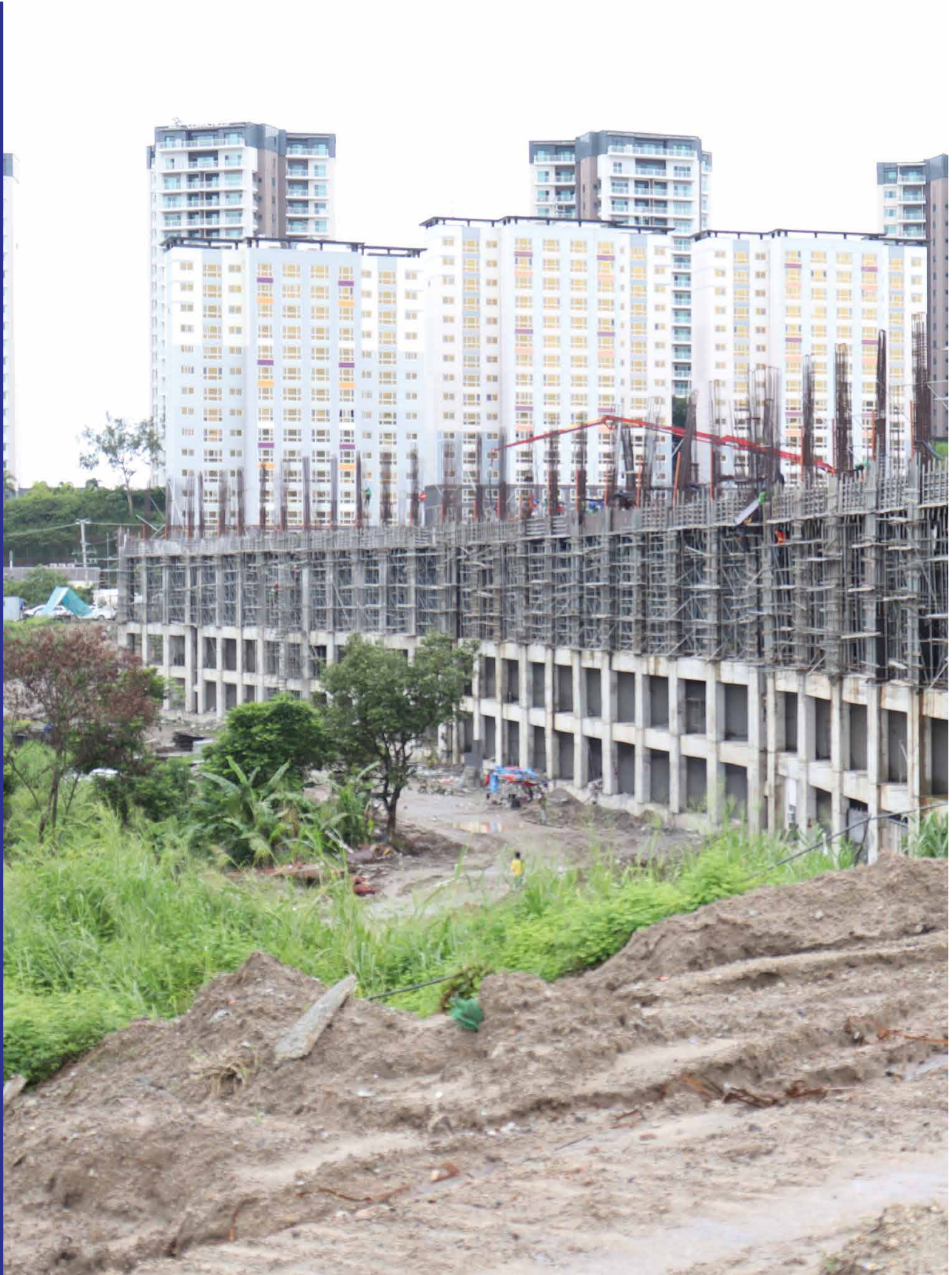
Work is already underway on an expansion of the existing casino and hotel space.
